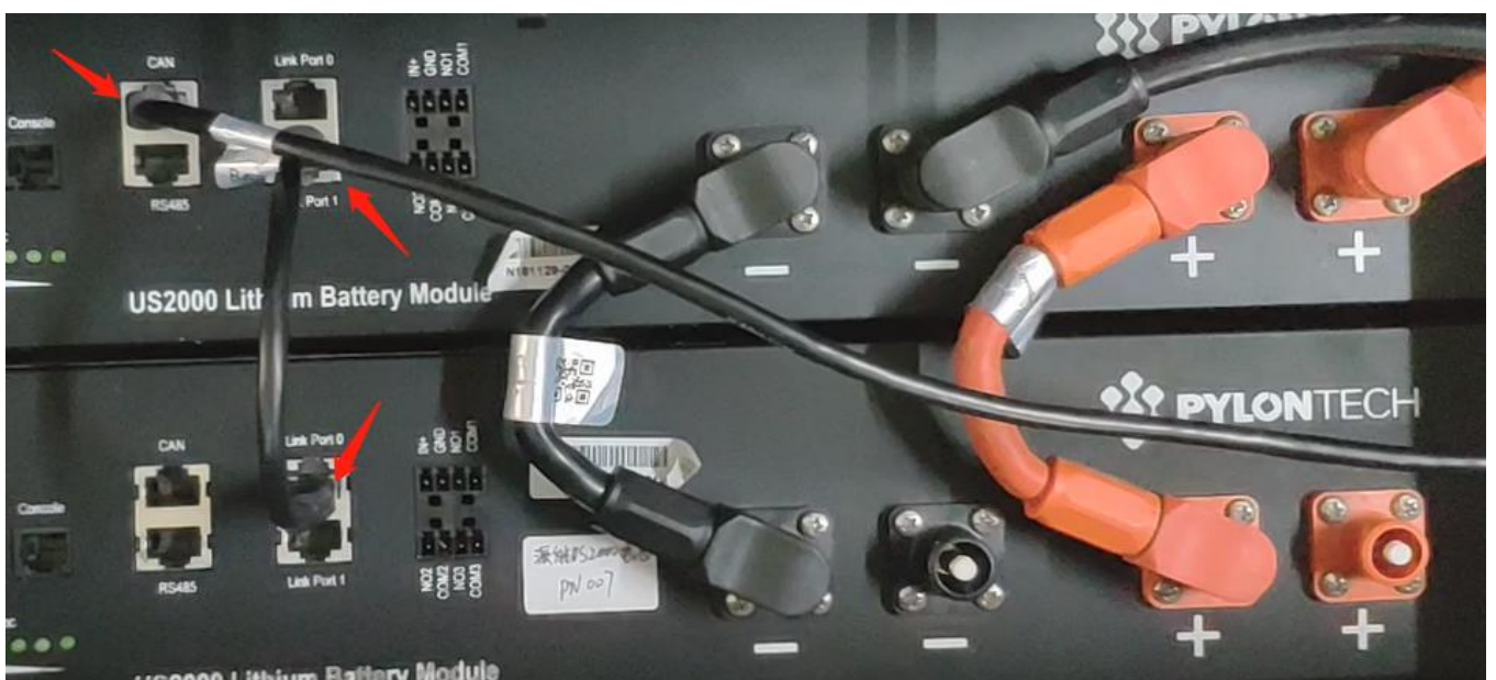
Figure1 .parallel connection of two batteries
